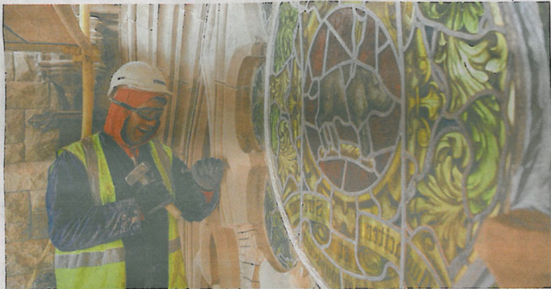
A stonemason at work on the large-scale overhaul of Derry's Guildhall. Photo: Lorcan Doherty
